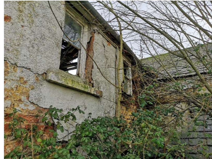
Fig2: Building Condition (Author, 2021)
