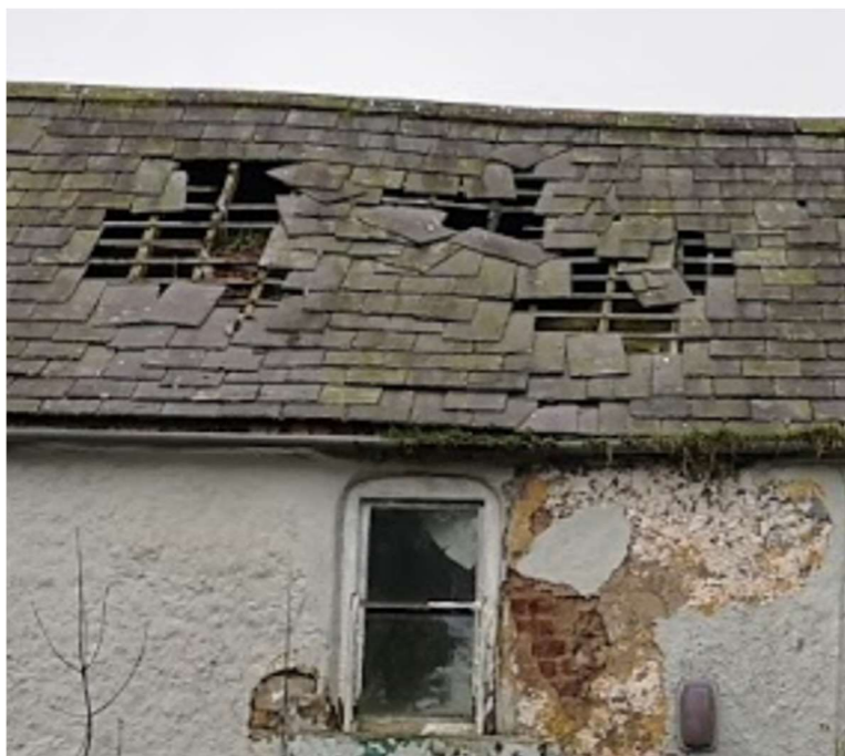
Fig65: Roof Condition (Author, 2021)
