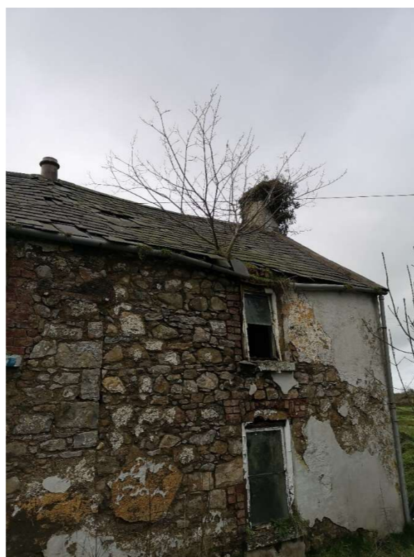
Fig57: Roof Condition (Author, 2021)
