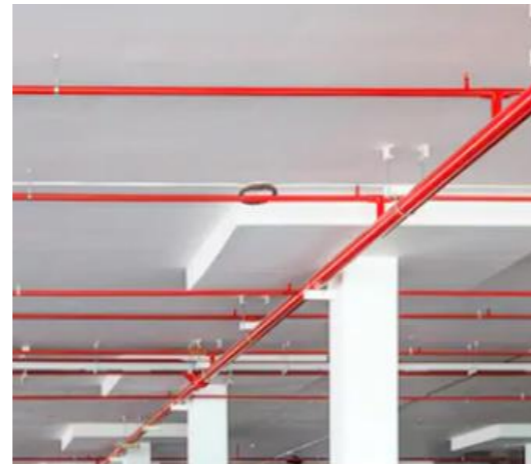
Fig13 - Fire Sprinklers (Service Master,
